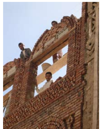
Figure 4: Brick arches and detailing applied as veneer on a concrete block wall.
